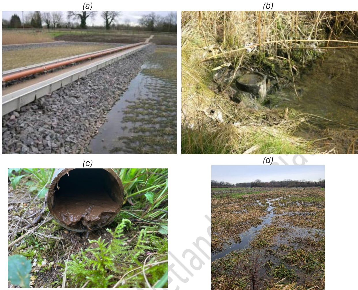
Figure 3.2 Examples of (a) good influent distribution on HF bed, (b) lack of maintenance of inlet riser pipes, (c) inlet pipe with sludge accumulation, (d) preferential flows developed as result of poor influent distribution in surface flow tertiary system. Credit: (a), (b), and (d) NbS Future/G Dotro, (c) Andy Freeman/ARM.
