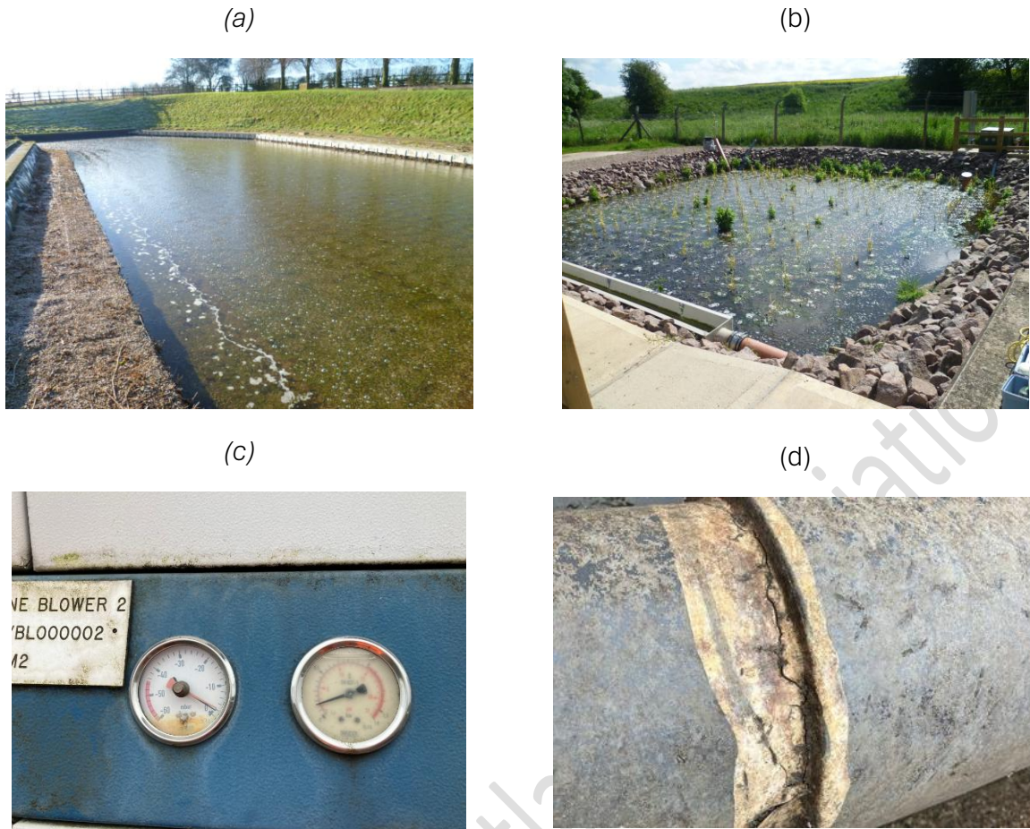
Figure 3.8 Aeration bubble patterns in new systems (a) uneven air distribution, (b) even bubble pattern, (c) Pressure gauge check on PD blower in need of maintenance (d) Aeration manifold leak. Photo credits: (a) and (b) NbS Future/G Dotro, (c) ad (d) ARM.
